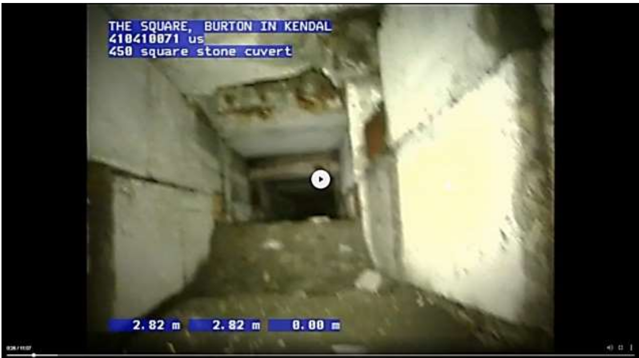
Figure 13: The combined sewer under Main Street crosses the culvert within the culvert barrel taking up approximately the bottom 150mm of the 450mm x 450mm culvert cross section.
