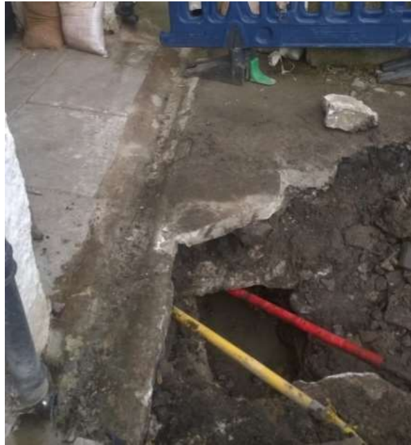
Figure 14 (right): Electricity cables in exposed culvert on 1/11/2017. Hole in the wall dropping onto the watercourse is visible behind barrier.
