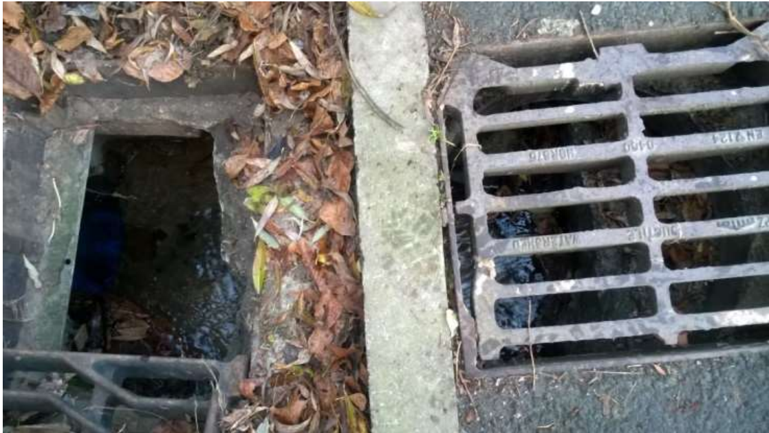
Figure 20: Photo of double gully arrangement on Tanpits Lane.
