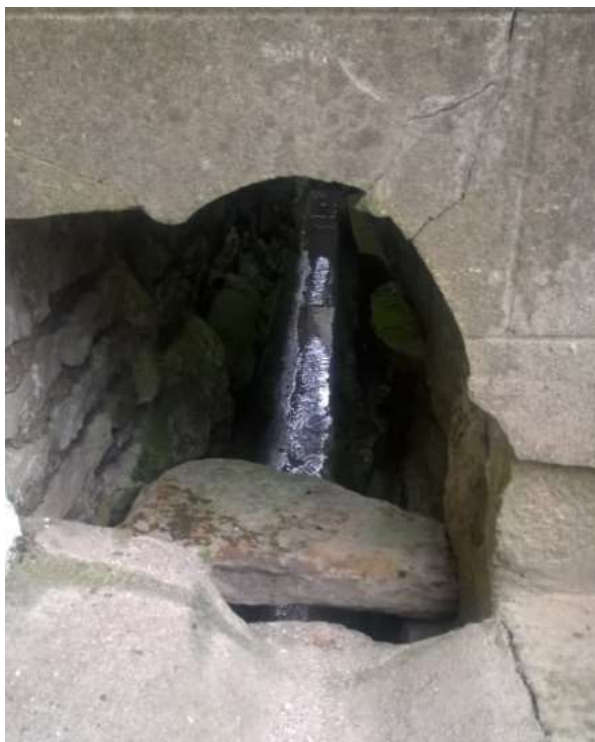
Figure 15 Hole in the wall dropping onto the watercourse.
