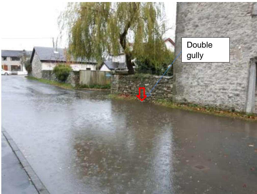
Figure 19: Photo of the flooding on Tanpits Lane outside The Tannery. Location of double gully arrangement on culvert is indicated by red arrow.
