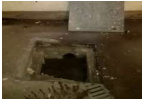
Figure 9: Cellar drain leading to manhole with a deeper drainage outlet which is below the level of the culvert so it is thought to lead to a soakaway.
